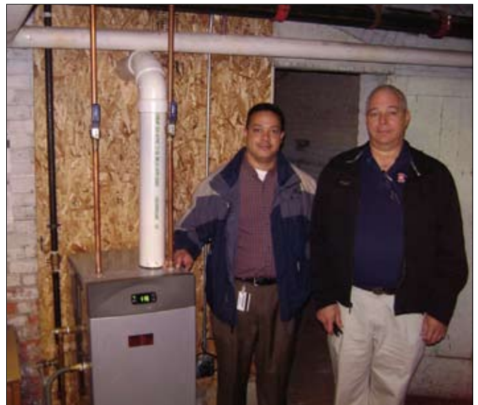
Rick Gerena (l) and Dan Gross chose the Eternal Hybrid Water Heater for its energy efficiency, environmental friendliness and lowered project cost.
